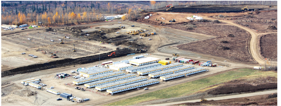
This aerial photo shows site preparations now underway for the Site C dam and hydroelectric generating station on the Peace River in northeast B.C. This is the first step in an almost decade-long construction period for Site C.
